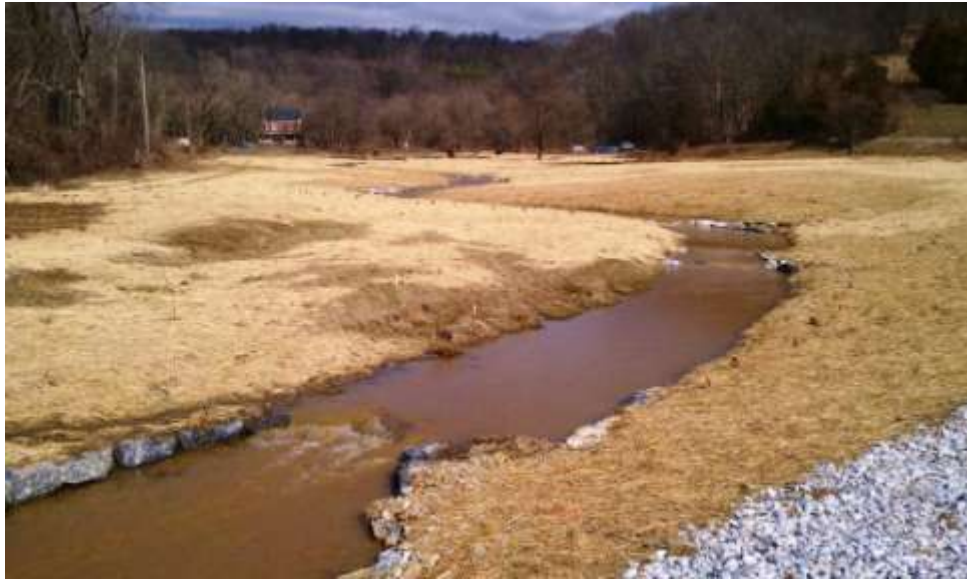
Natural Stream Channel Design stream Restoration on Pine Run, North Branch Muddy Creek
