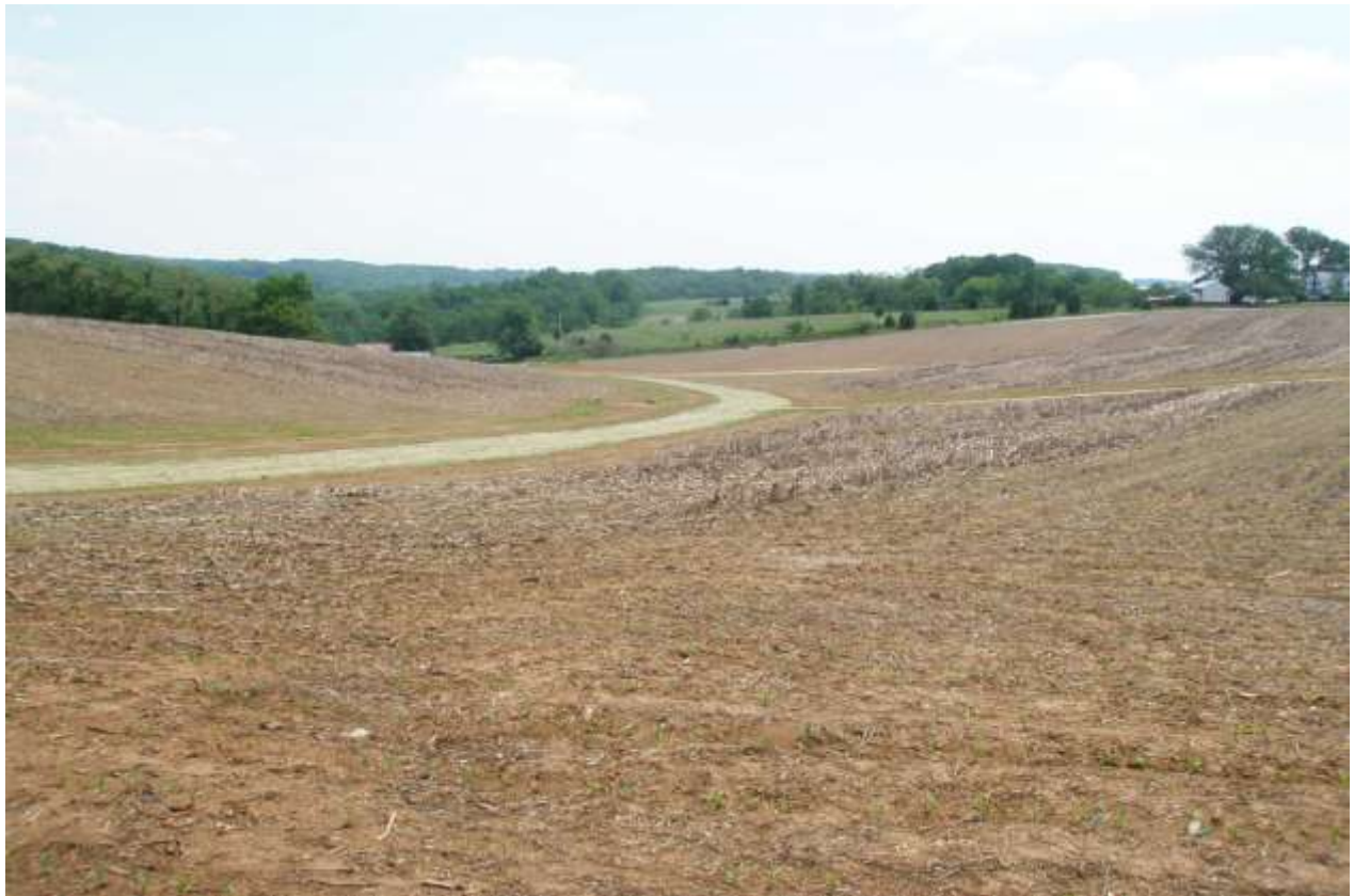
Grass waterways installed at the Adam Shearer farm in Lower Chanceford Township- Muddy Creek Watershed
