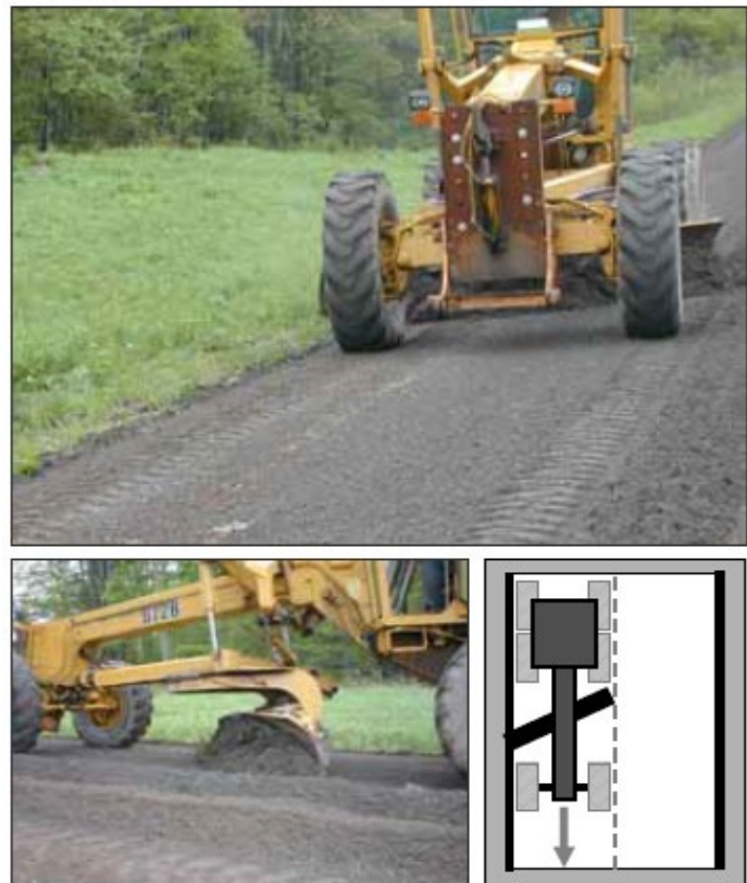
Figure 25. Large aggregate that has accumulated on the shoulder is pulled to the center of the road and mixed with fine aggregate particles as it rides up the blade. The blended aggregate is deposited in a wind-row in the center of the road. Note the high moisture content of the graded material.
