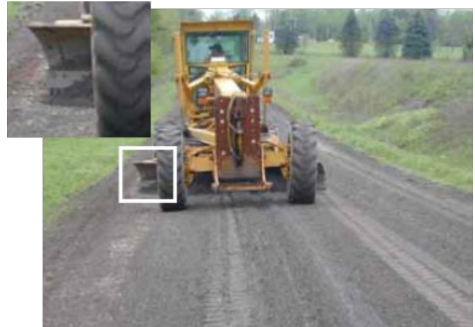
Figure 31. Grader grooming the road. Notice the grader blade is not carrying a lot of material.
