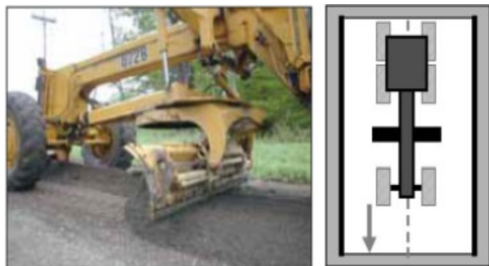
Figure 30. Grader leaving the road with a high flat center.
