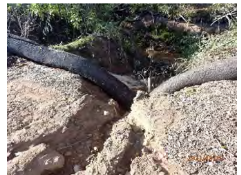
Above: Compost filter sock undermined by runoff observed during a routine site inspection.
