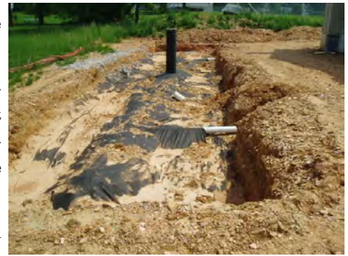
Above: An underground seepage pit on a residential lot that has not yet been back-filled and is clogging with sediment from surrounding disturbed areas.
